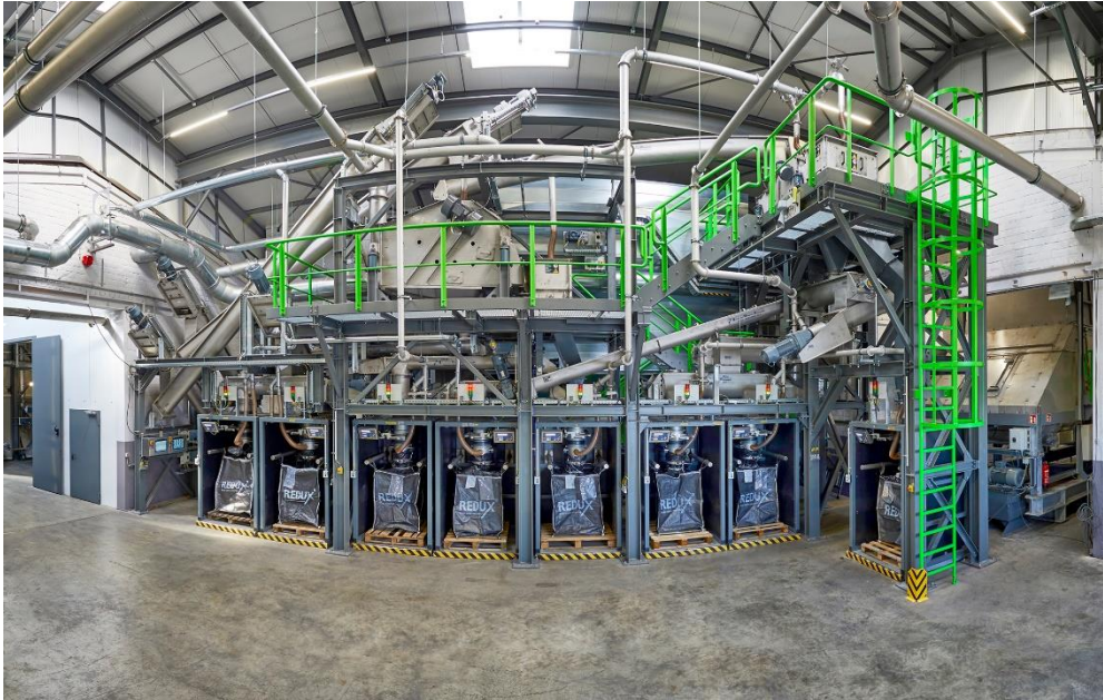
Photo 1: R: Recycling plan for all types of lithium batteries in Bremerhaven. Photograph rights: Saubermacher.
