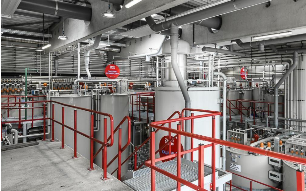
Internal view of the chemical/physical treatment plant; photo credit: Saubermacher/Pixelmaker
